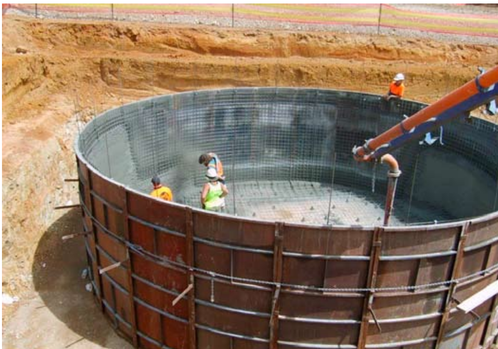
A large underground water storage tank being installed at an ACT public school.
